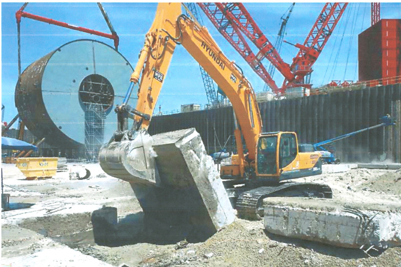
Cut sections were lifted from the slab by excavators and moved to the dock wall for removal by crane.
