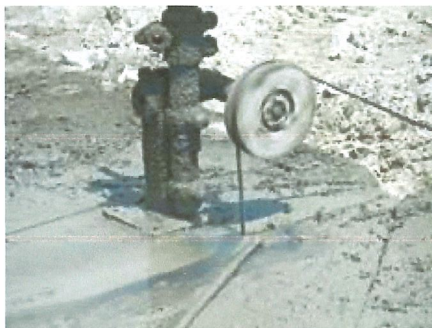
Wire saws were used to cut 10-foot square sections that were 36 to 39 inches thick.
