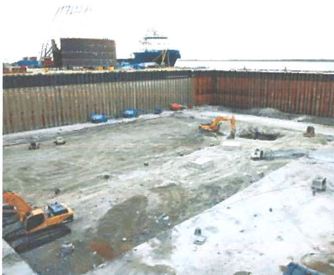
The damaged graving dock measured 600 feet long and 250 feet wide.
